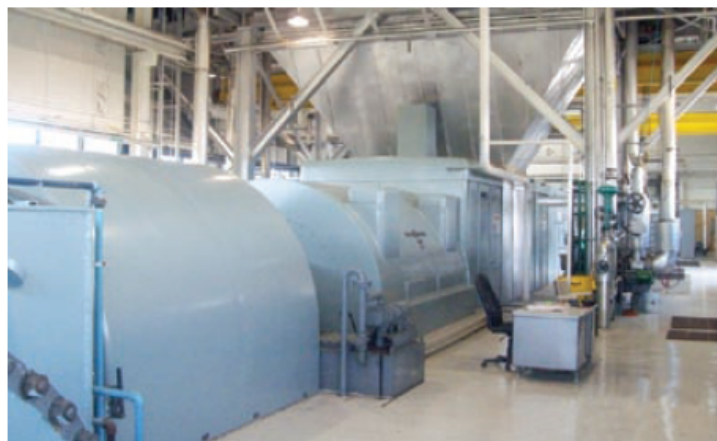
B. Wolverine Power Supply Cooperative Inc's STAG 105 looks almost new after 41 years of service. Moving from left to right: steam turbine, generator, load gear, vertical exhaust transition from the gas turbine to the heat-recovery steam generator and stack, and the GT package further down. Bolted flange in lower left-hand corner is part of the condenser
